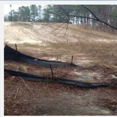
Failing Silt Fence
