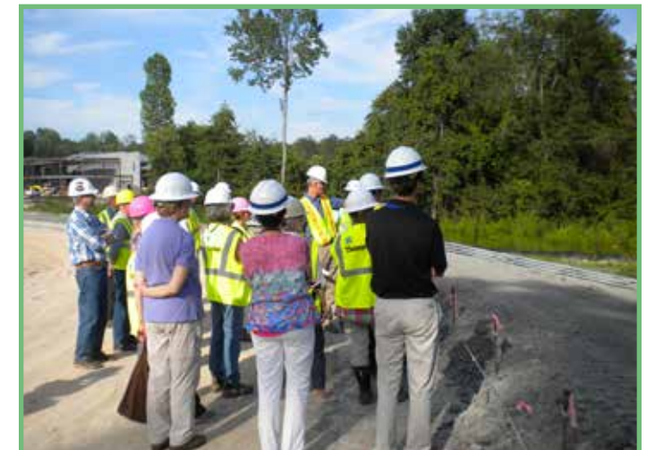
Tour of the Richland County District 2 Elementary 20 construction site near the confluence of Little Jackson Creek and Jackson Creek.
