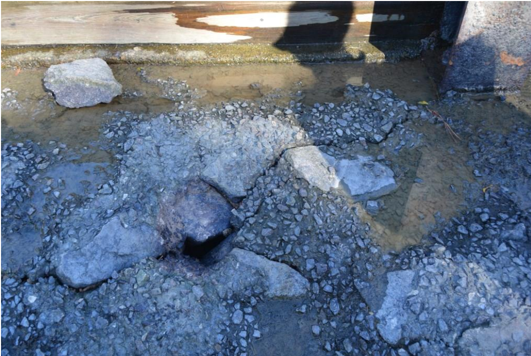
Photo 8: Voids and cracks in concrete/rockfill overflow spillway surface
