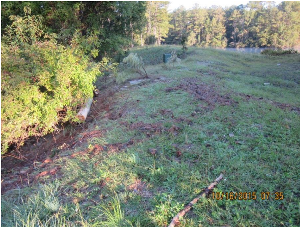
Photo 4: Woody growth on the left downstream slope
