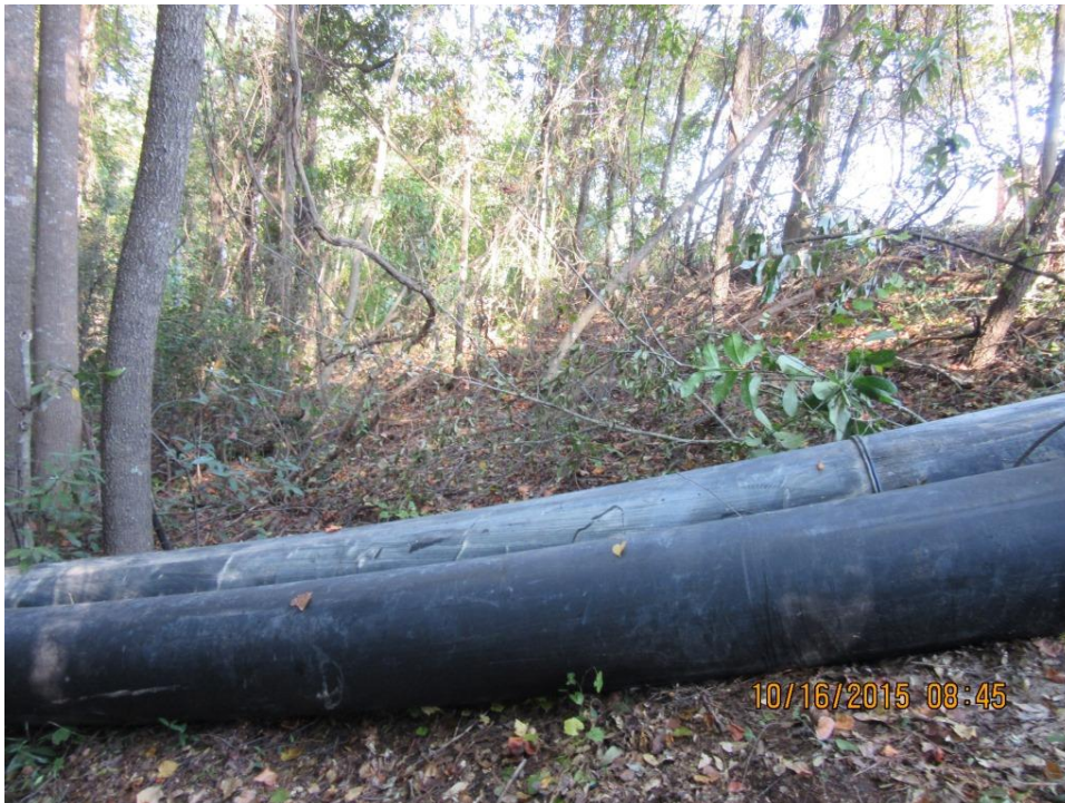
Photo 6: Tree growth on downstream slope of embankment; temporary pump discharge pipes are in the foreground
