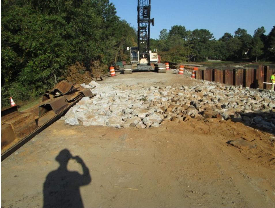
Photo 3: Sinkhole area on embankment crest showing temporary rock fill
