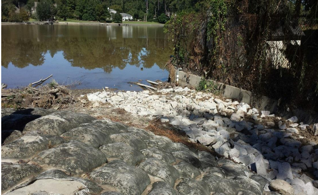
Photo 7: Approach to auxiliary concrete-chute spillway showing temporary rockfill repair of scour
