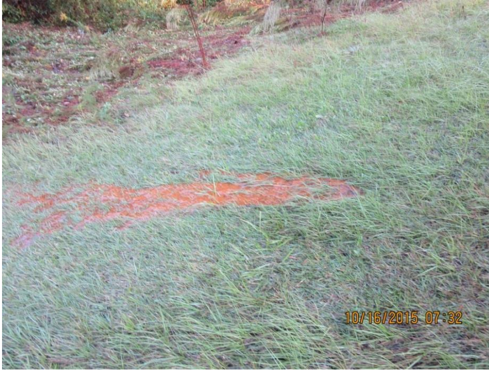
Photo 9: Seepage at downstream end of auxiliary spillway
