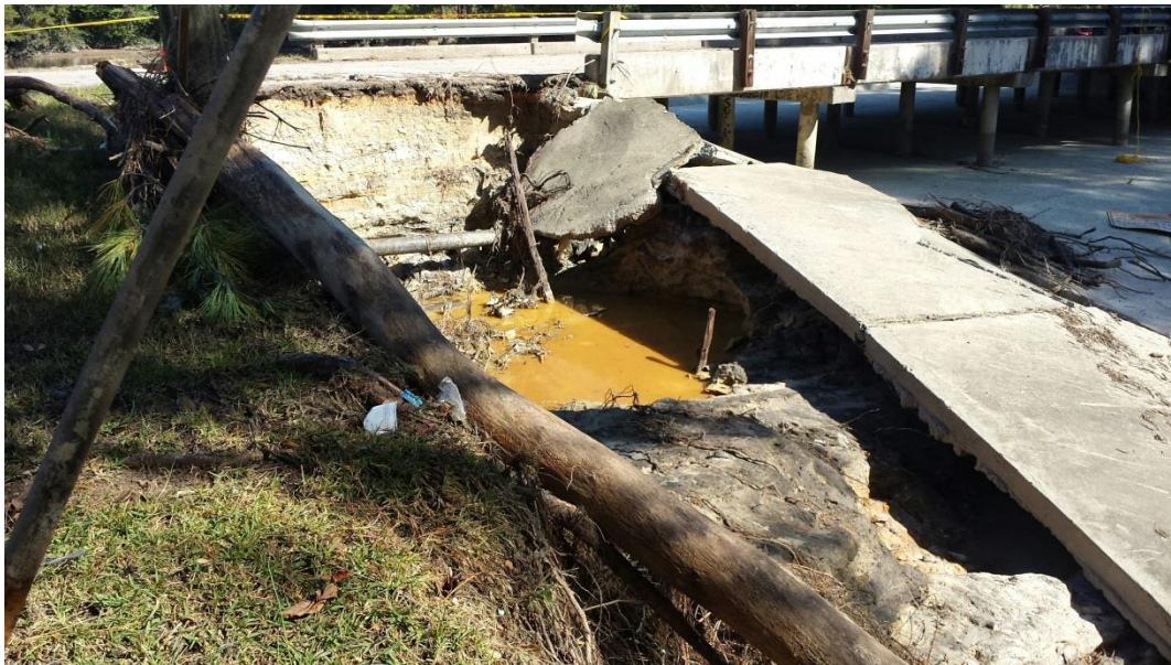
Photo 8: Erosion of concrete of auxiliary spillway adjacent to embankment
