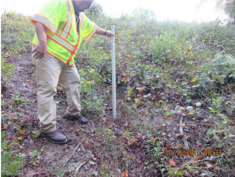
Photo 7: Erosion on the downstream slope of the embankment
