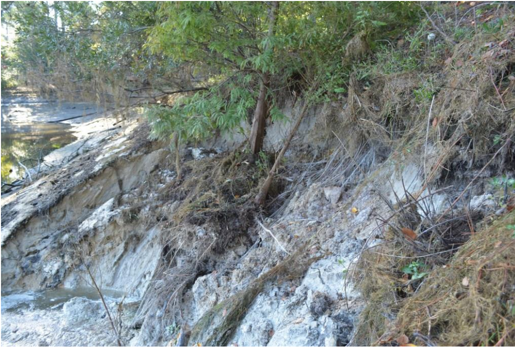
Photo 4: Upstream embankment slope failure
