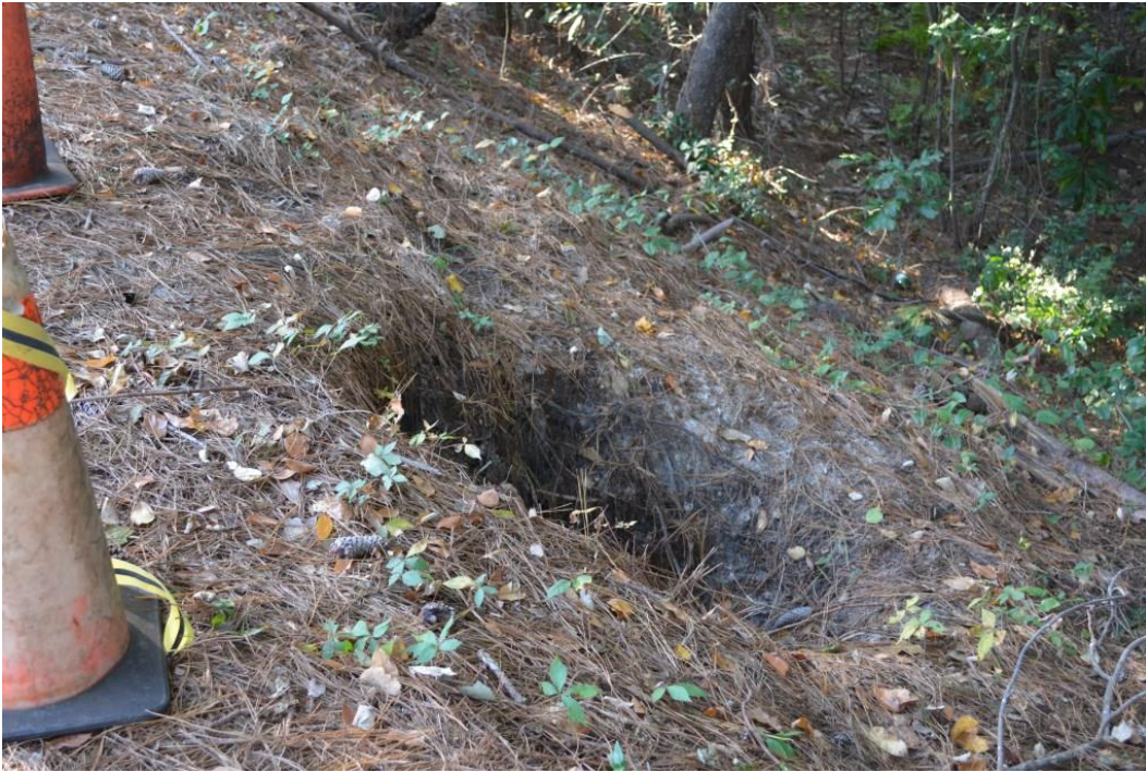
Photo 8: Depression on downstream slope above spillway alignment
