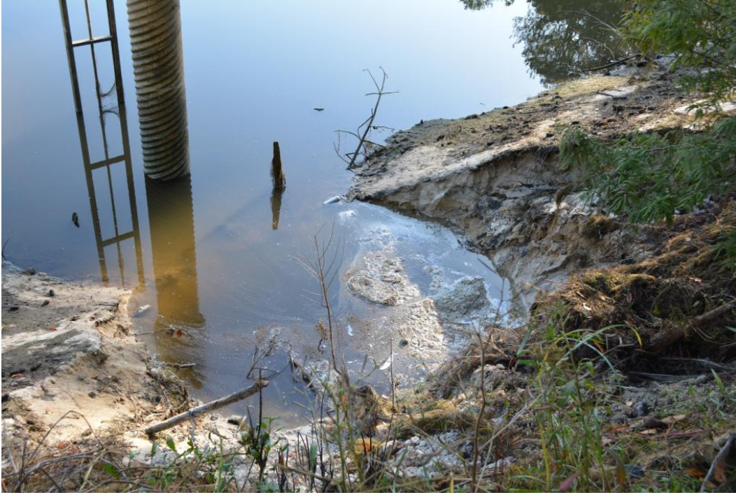
Photo 7: Upstream slope failure along service spillway alignment
