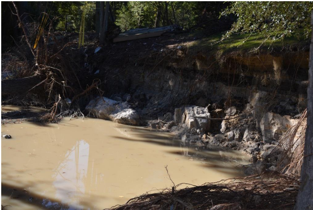
Photo 2: Eroded downstream face of embankment dam
