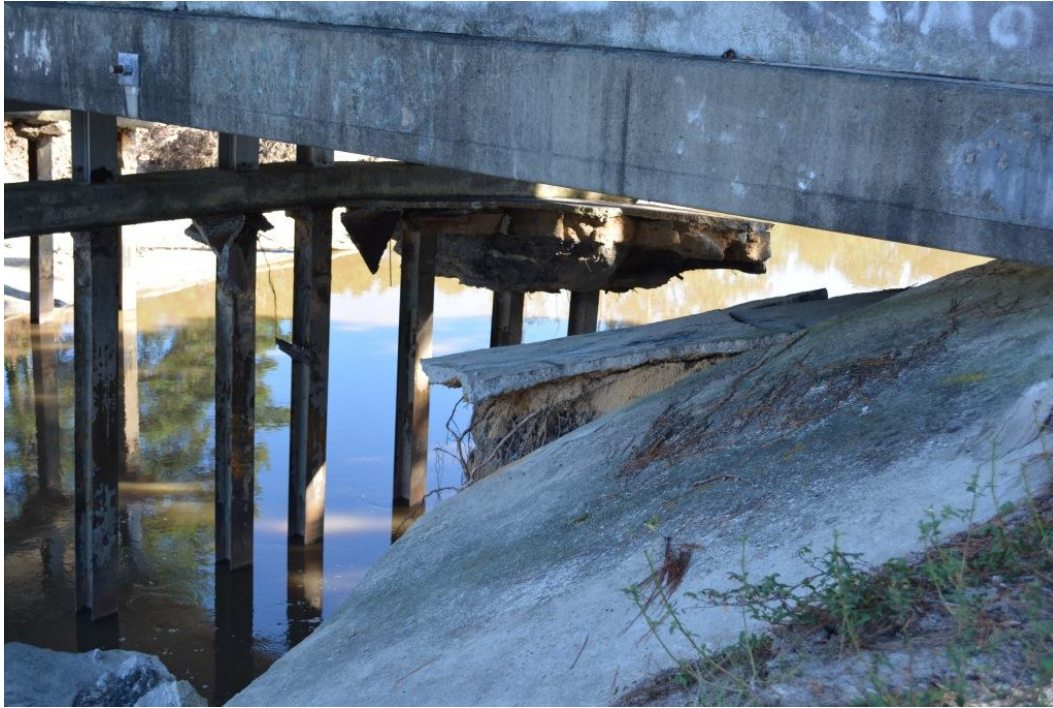
Photo 5: View of eroded auxiliary spillway area beneath the bridge
