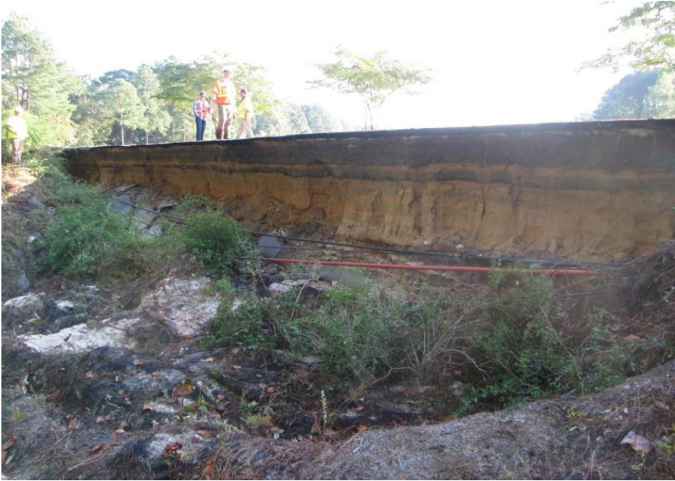
Photo 3: Downstream embankment slope failure along alignment of service spillway low-level outlet
