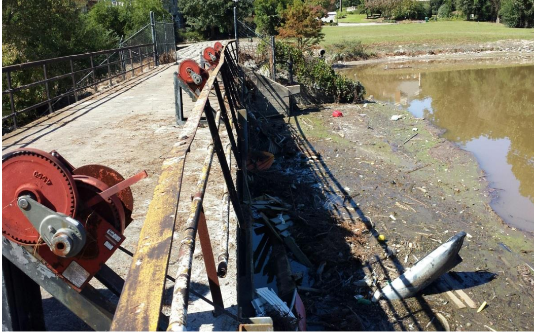
Photo 5: Damaged guard rail obstructing crest gate winch operators
