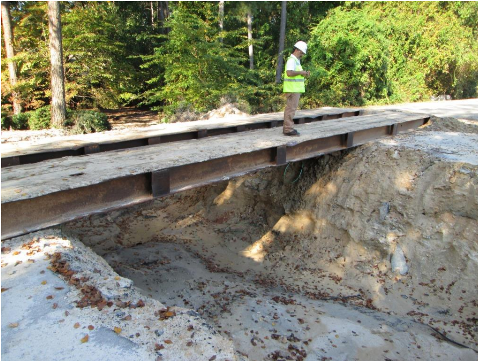
Photo 2: Temporary trench excavated to function as an emergency channel near the left abutment
