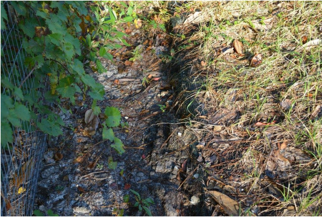
Photo 4: Erosion on downstream slope
