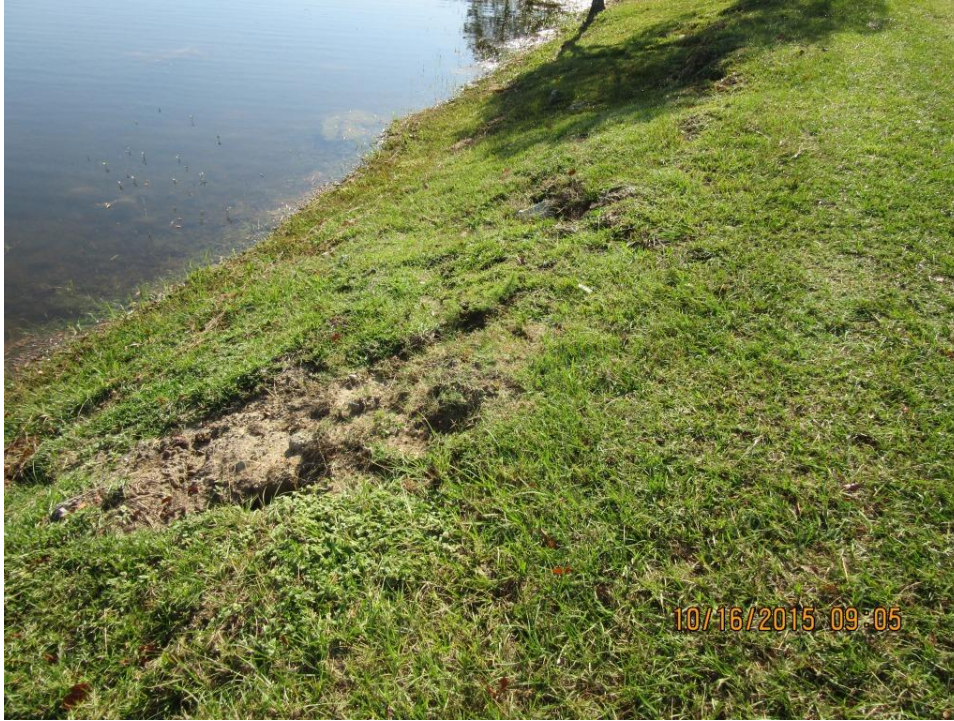
Photo 3: Slough on upstream slope of the embankment dam
