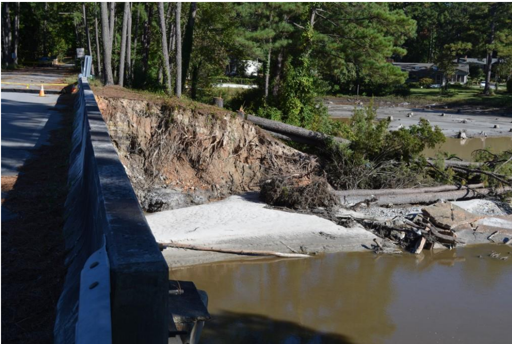
Photo 2: View of eroded embankment at left abutment of the auxiliary spillway looking downstream
