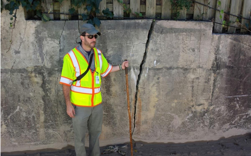
Photo 10: Crack in left wall of auxiliary spillway.
