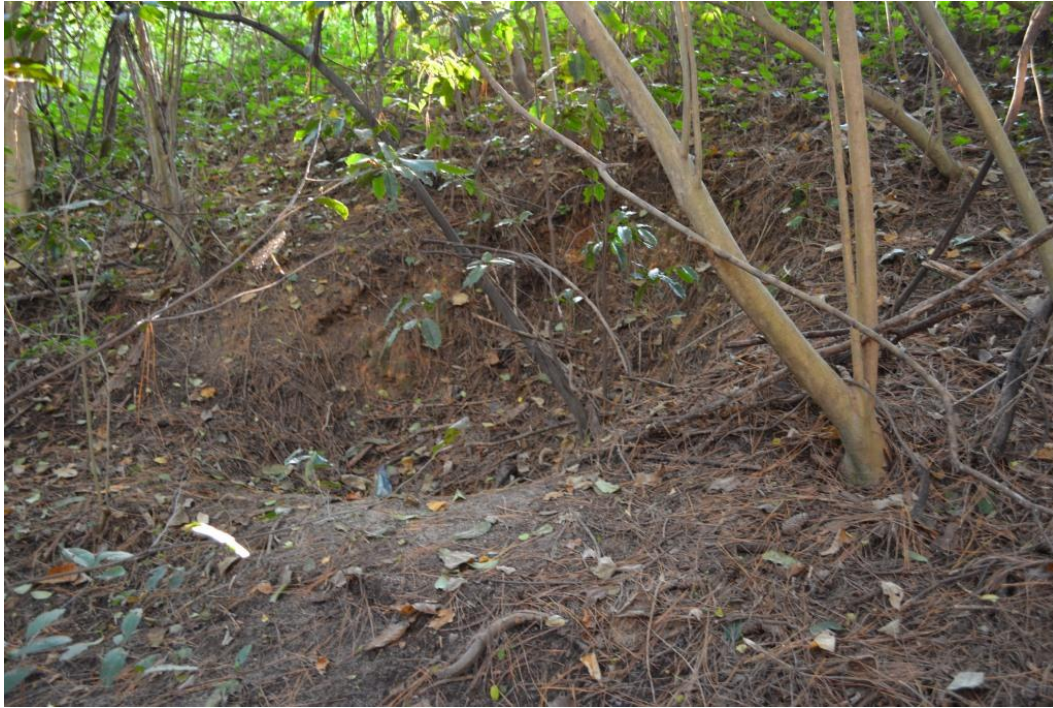
Photo 7: Depression on downstream face above principal outlet pipe
