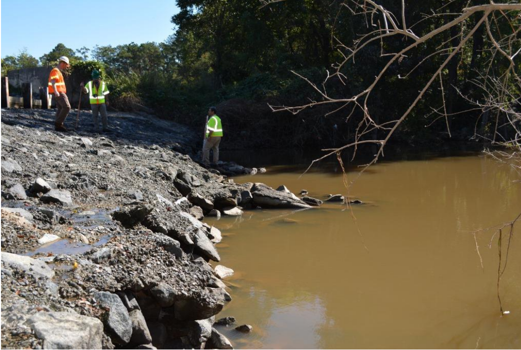
Photo 7: Toe of concrete/rockfill overflow spillway; outlet pipe of service spillway submerged at toe of spillway
