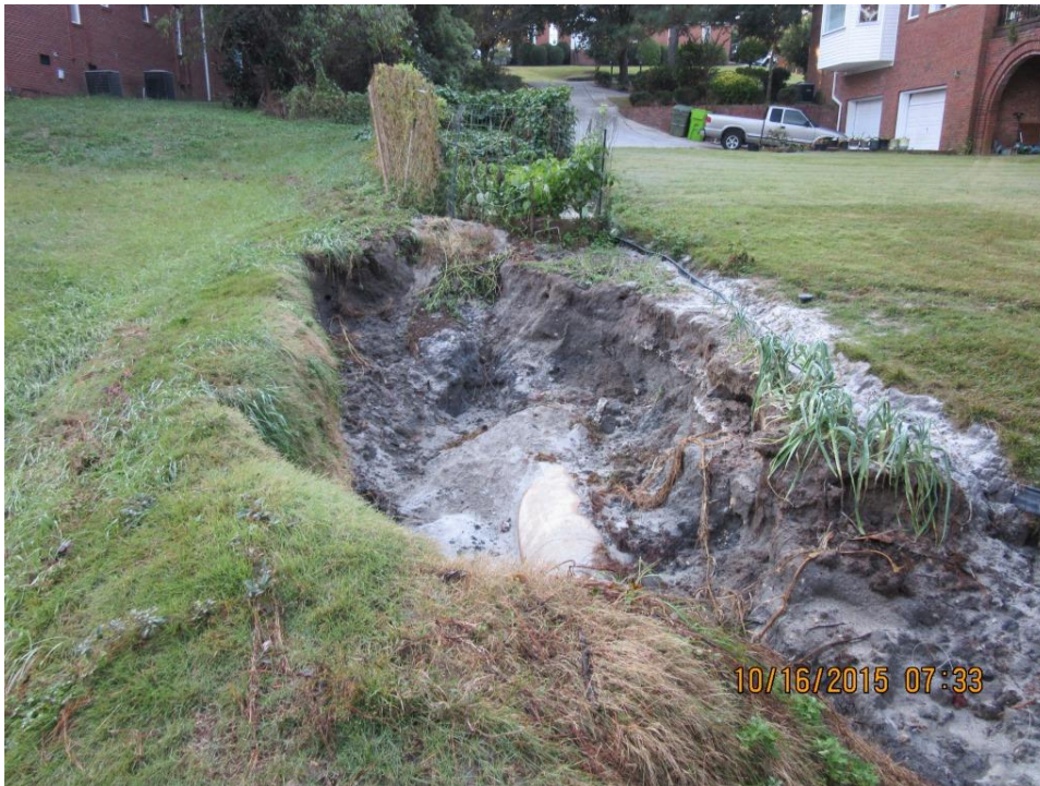
Photo 10: Eroded area at downstream end of auxiliary exposing RCP pipe, presumably a stormwater main
