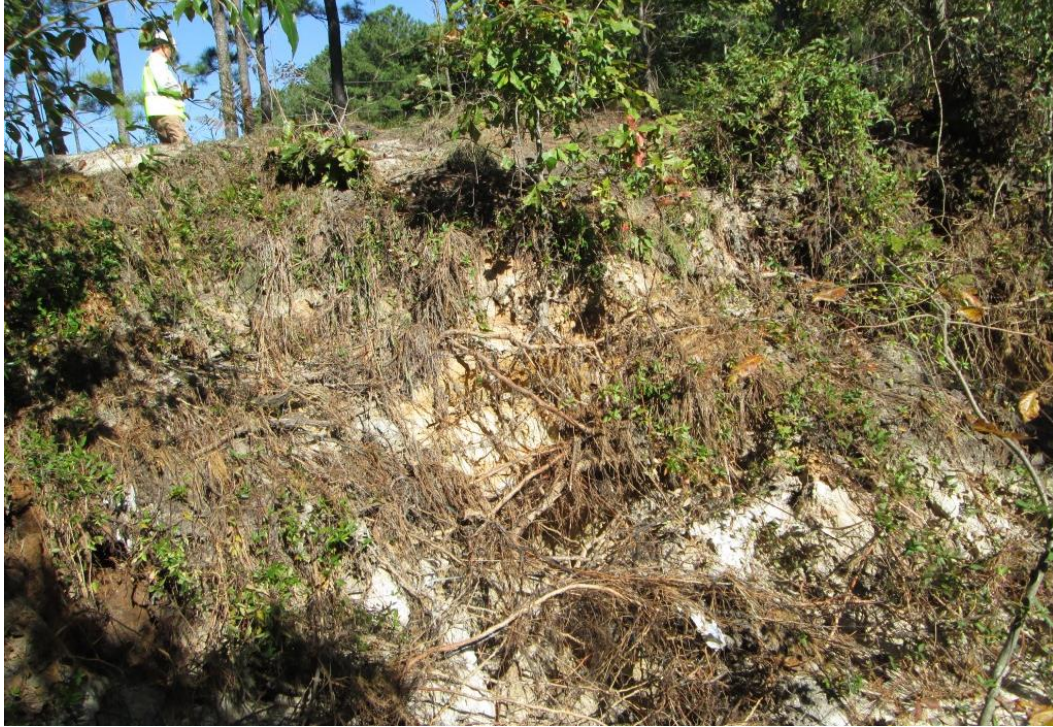
Photo 3: Significant erosion and undercutting of downstream slope of embankment resulting in a near-vertical slope maintained by root systems.
