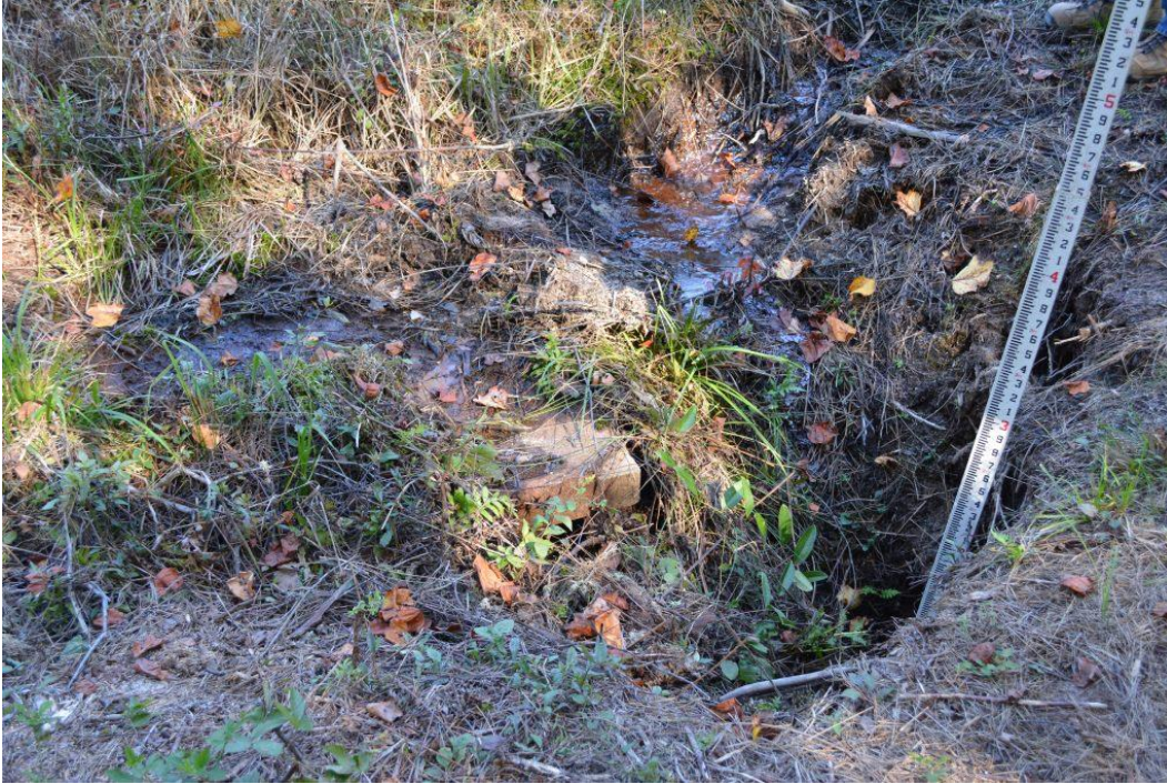
Photo 5: Hole adjacent to catch basin at toe of embankment
