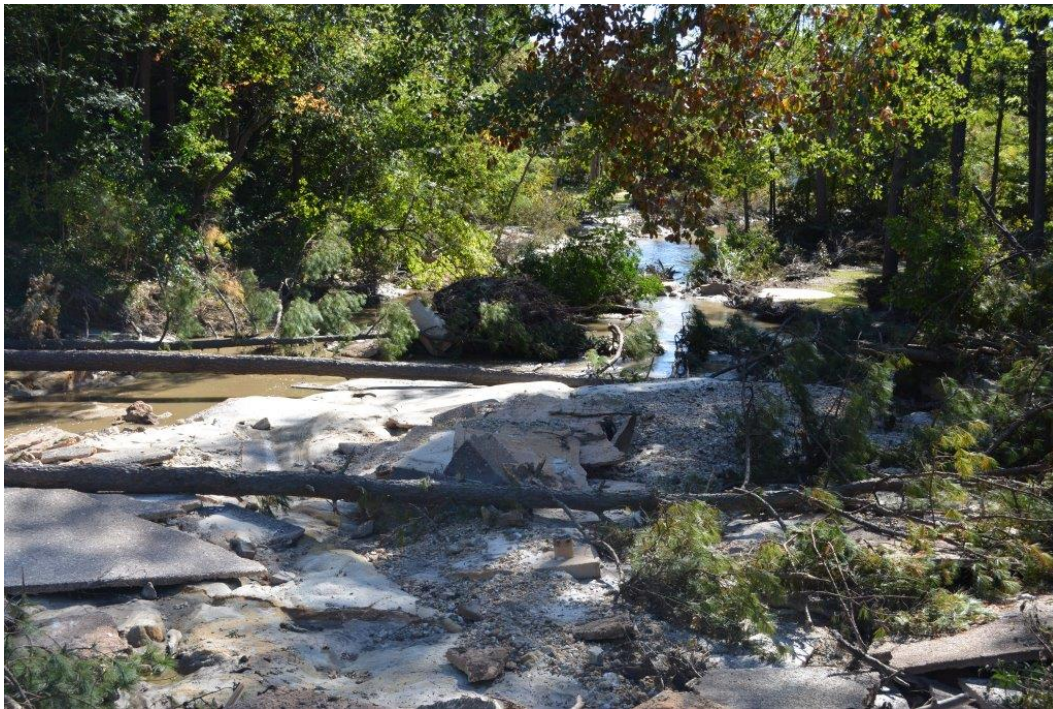
Photo 6: View of the auxiliary spillway looking downstream of bridge; concrete debris is seen in the foreground
