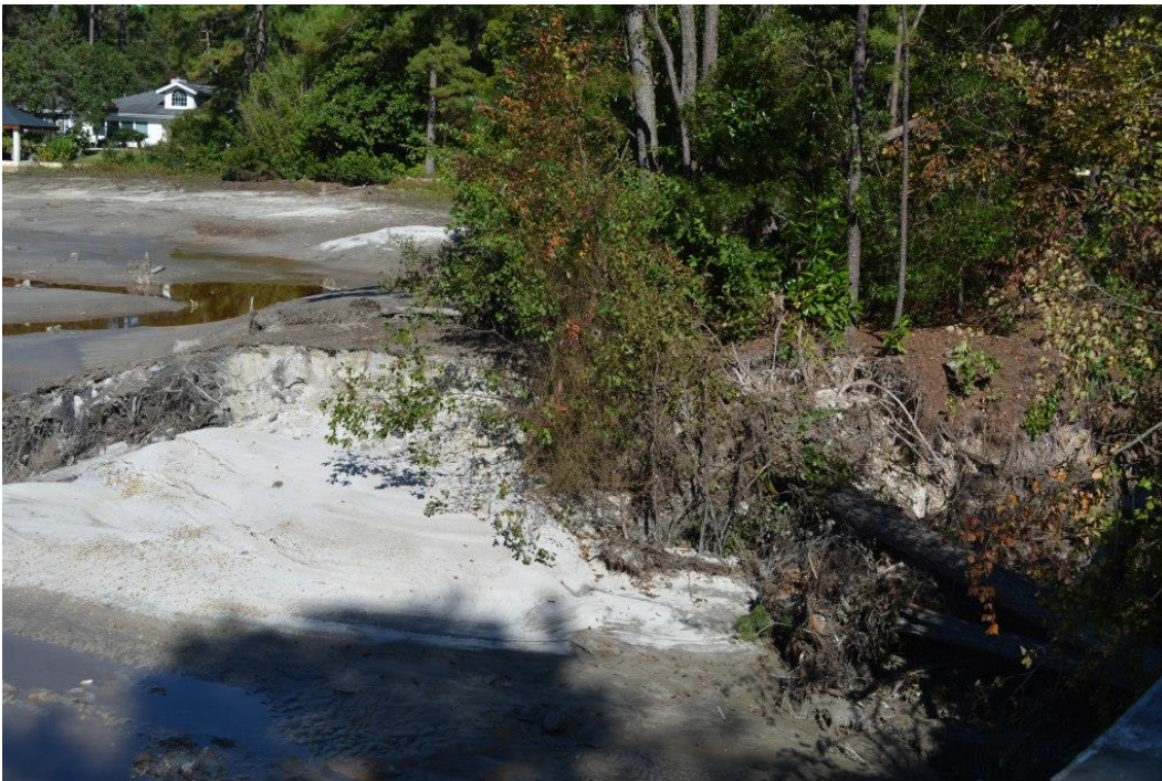
Photo 2: Erosion along the left side of approach channel to the auxiliary spillway
