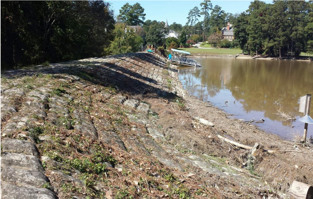
Photo 1: View of crest and upstream slope of armored left embankment dam looking from the left abutment
