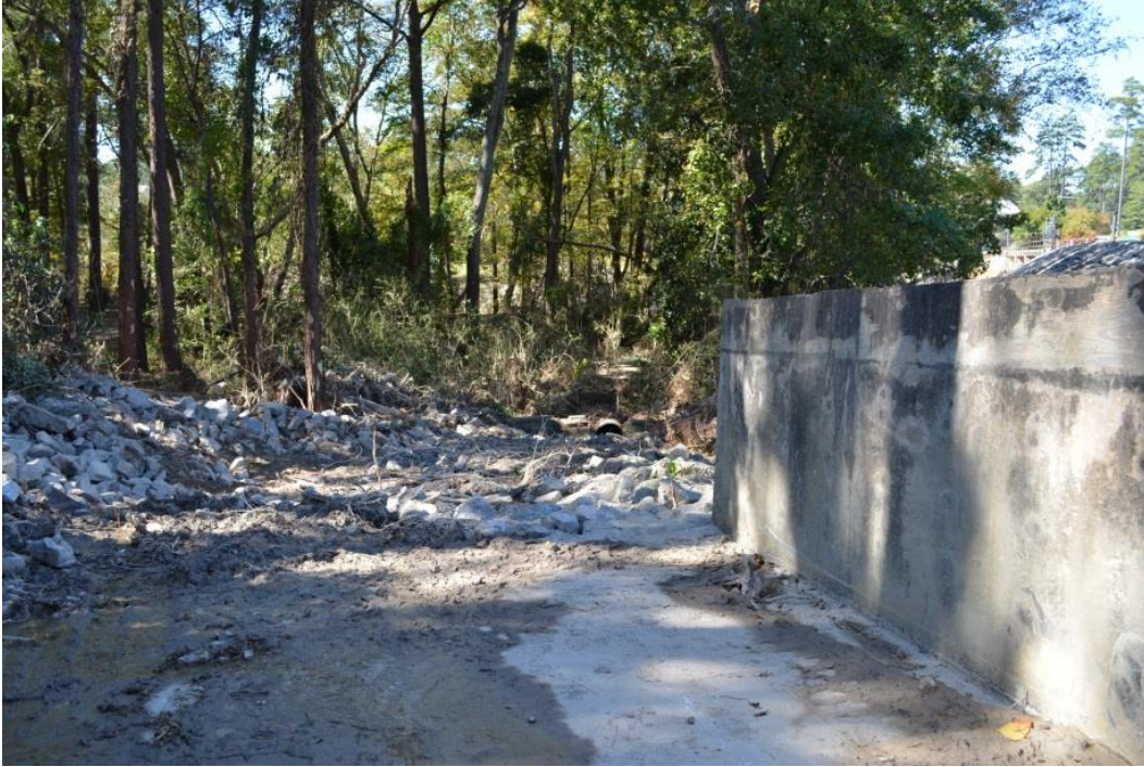
Photo 9: Downstream end of auxiliary spillway concrete chute with temporary rockfill of scour
