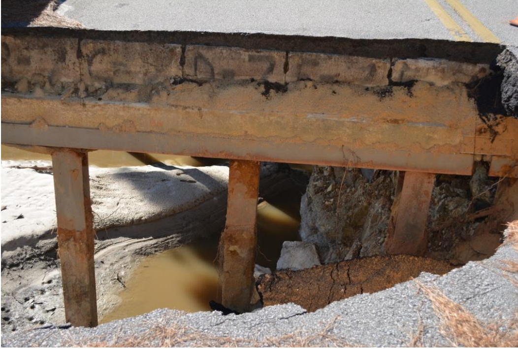
Photo 4: Erosion at bridge abutment
