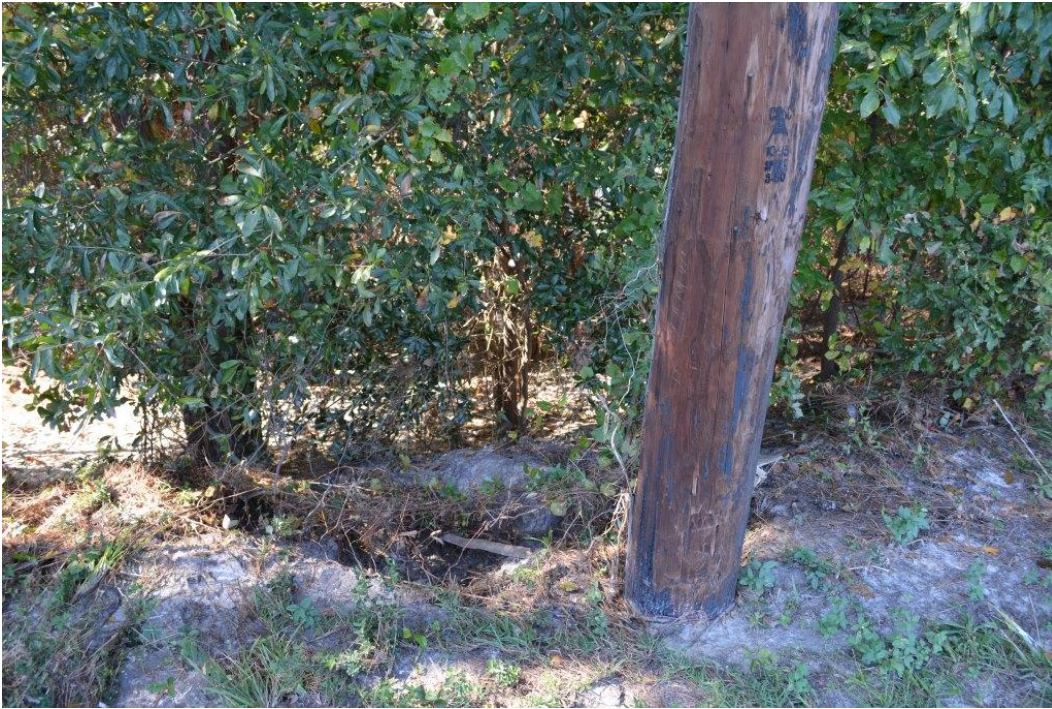
Photo 4: Slough and debris on downstream slope
