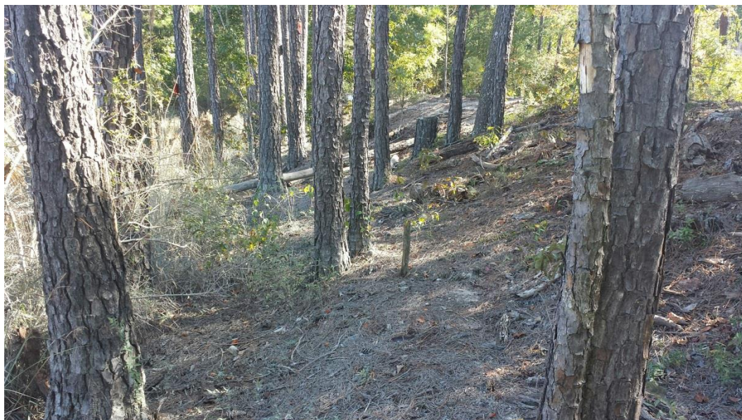
Photo 2: Tree growth on upstream embankment slope
