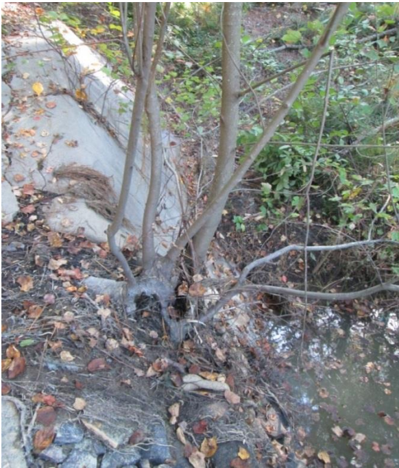
Photo 8: Tree growing in left abutment of the upper masonry stone dam
