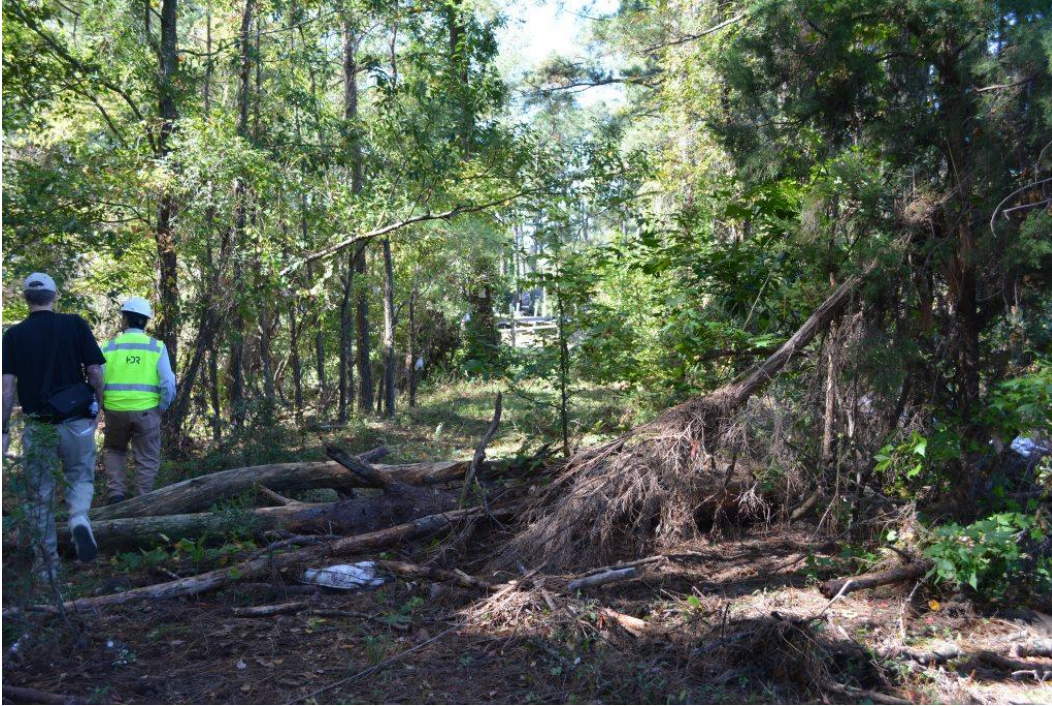
Photo 3: Right embankment crest looking toward right abutment showing tree growth on upstream and downstream slopes
