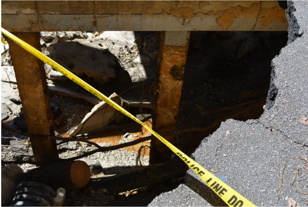
Photo 3: Area of auxiliary spillway wash-out at the left bridge abutment
