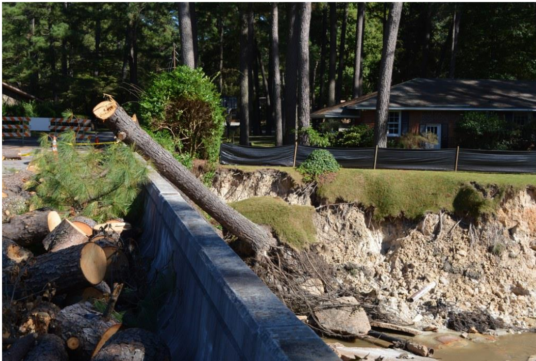
Photo 4: Erosion at the left abutment viewed from the bridge
