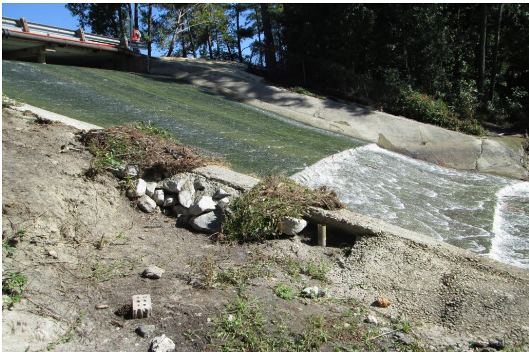
Photo 6: Eroded/filled areas along right side of auxiliary spillway channel
