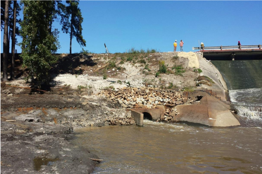
Photo 1: View of downstream slope of right embankment; note the void in concrete near the toe of the auxiliary spillway, and jute mat located adjacent to the bridge to stabilize an eroded area
