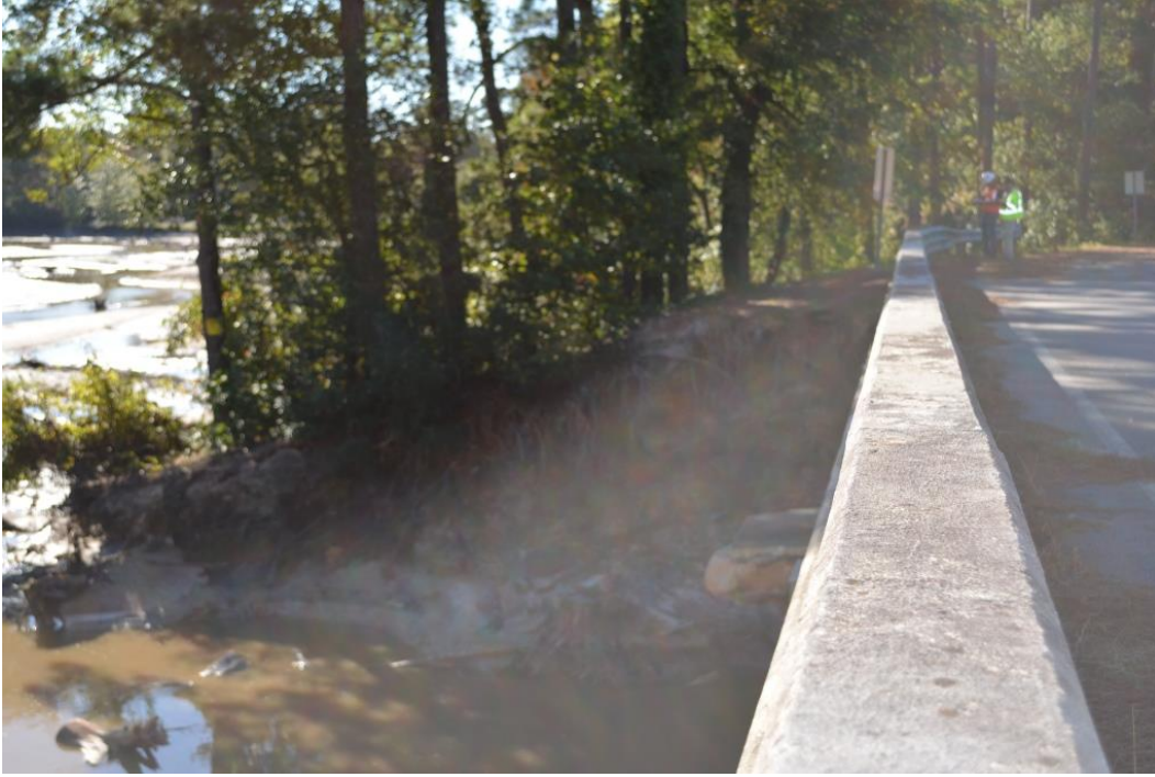
Photo 3: Erosion of embankment at the right abutment of the auxiliary spillway looking downstream
