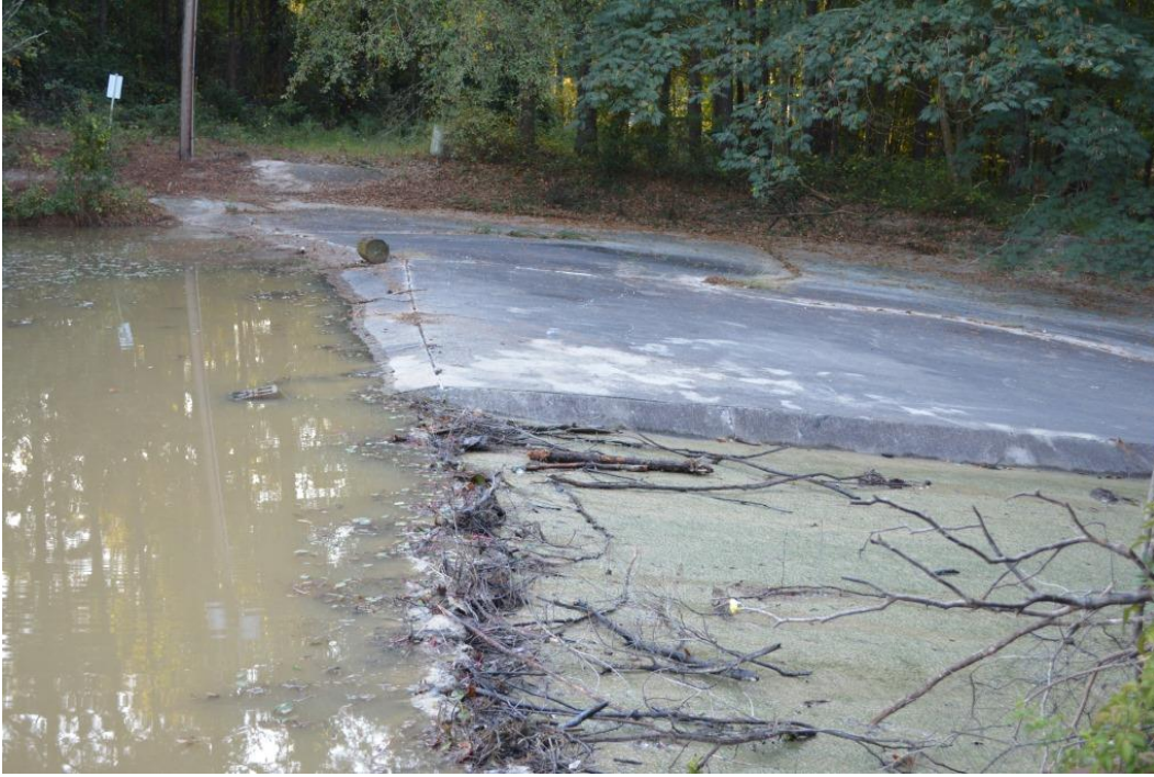
Photo 9: Auxiliary spillway with debris
