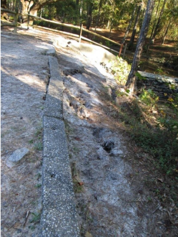
Photo 10: Right bank slump between upper and lower masonry stone dams
