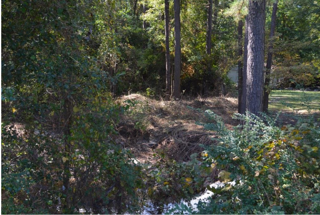
Photo 7: Erosion at plunge pool of auxiliary spillway no. 2
