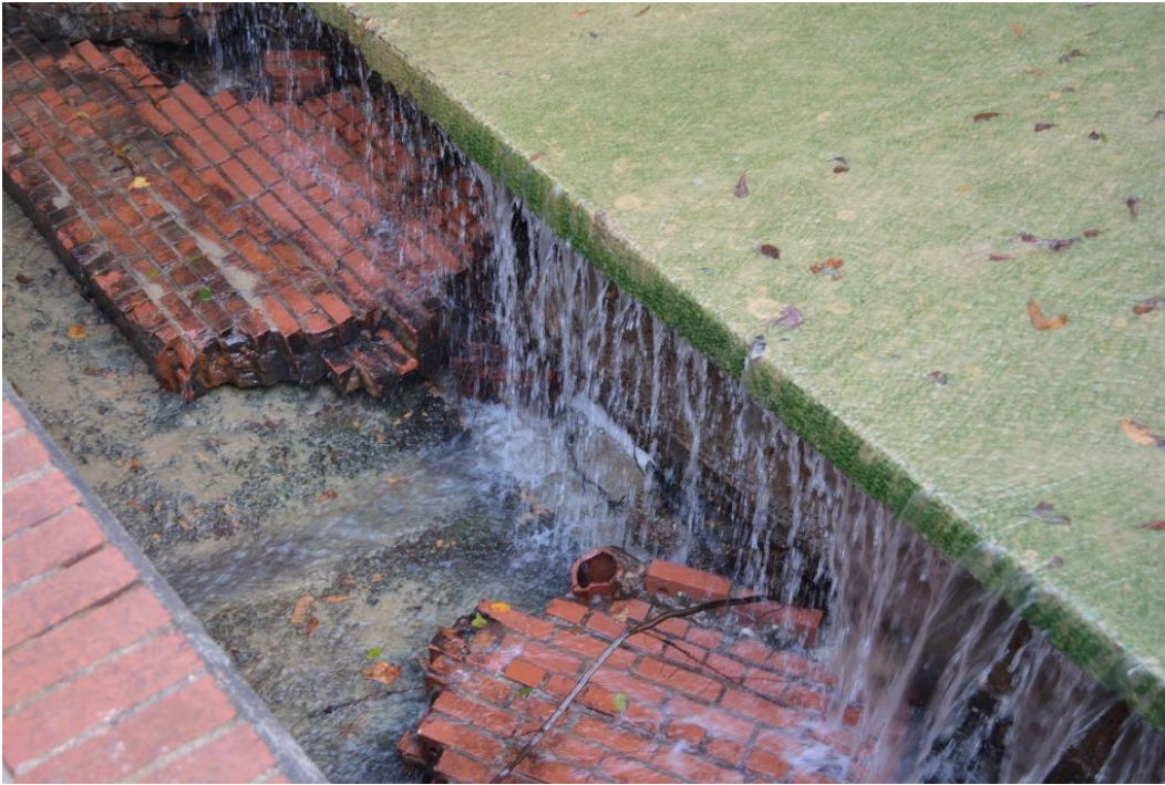
Photo 10: Damage at downstream end of auxiliary spillway
