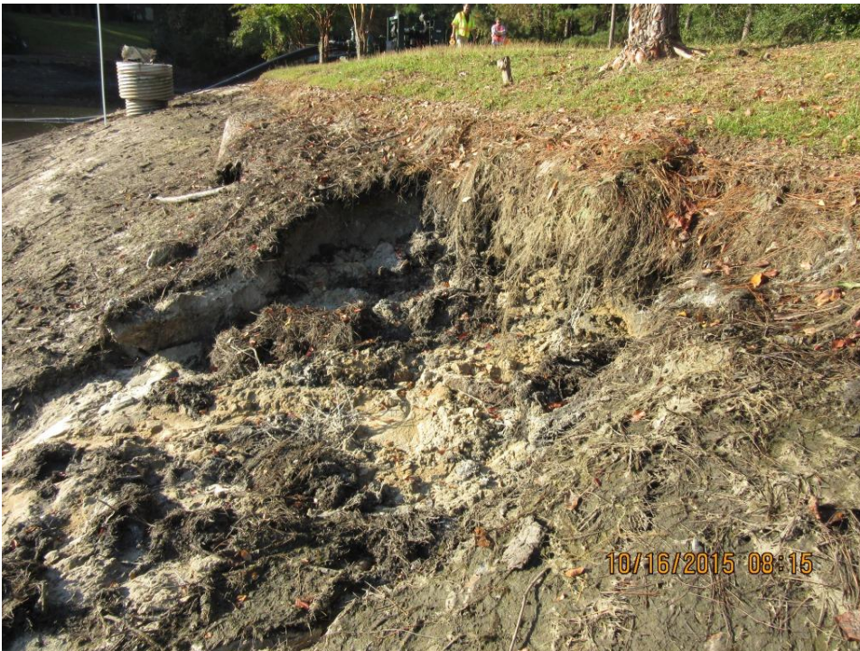
Photo 2: Upstream embankment slope slough
