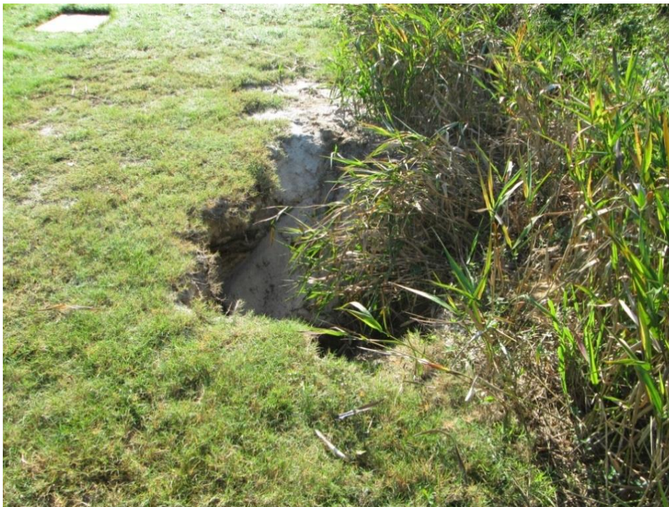
Photo 6: Erosion on downstream slope of embankment, approximately 30 feet upstream of the service spillway outlet
